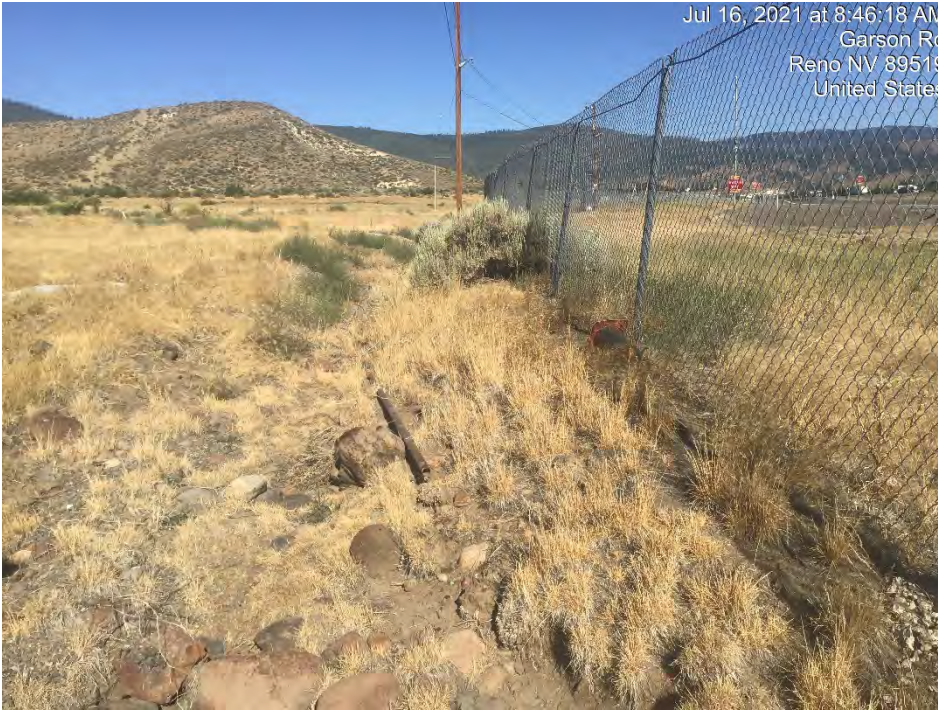
Photograph 25: Drainage area near fence by Highway 80 East. Photo facing west.
