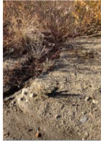
Photograph 34: Erosion sign from NDOT asphalt pad crossing dirt road and entering ditch; facing southwest (Image 0338)
