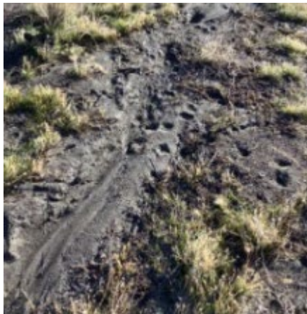
Photograph 19: Heavy sedimentation in swale bottom below rilling from I-80 (Image 0263)
