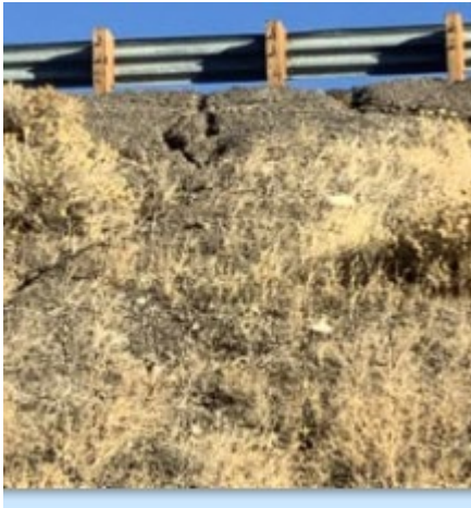
Photograph 5: Surface runoff from I-80 causing rilling and swale sedimentation (Image 0340)
