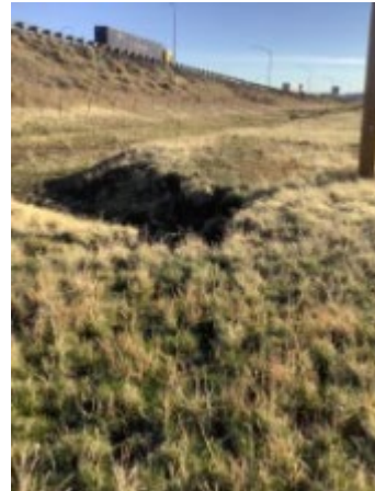
Photograph 6: Minor ditches and erosional features feeding into storm water swale (Image 0248)
