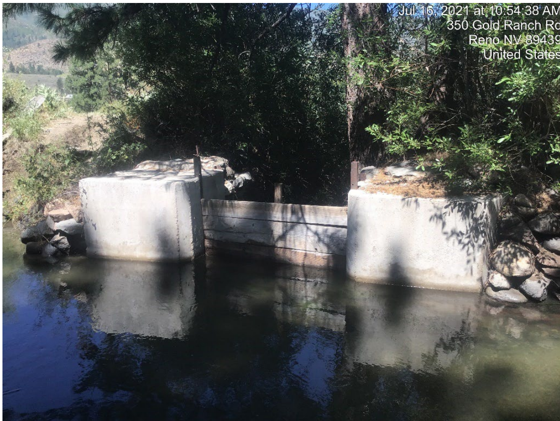
Figure 5 Steamboat Ditch Typical Natural Drainageway Flashboard Gate (outside of project area)
