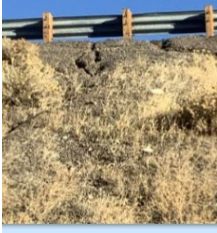
Photograph 5: Surface runoff from I-80 causing rilling and swale sedimentation (Image 0340)
