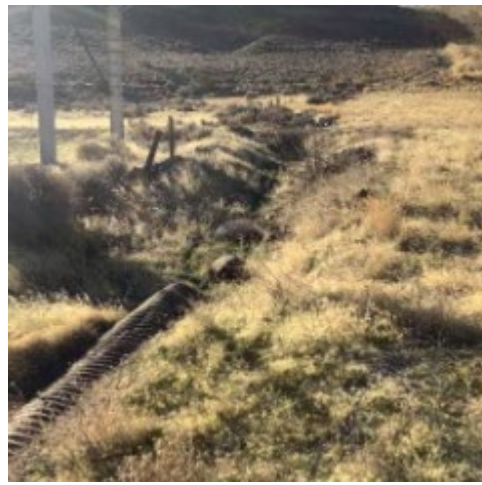
Photograph 18: Old water pipe and ditch just upslope from concrete foot and conveyance pipe; facing south (Image 0279)
