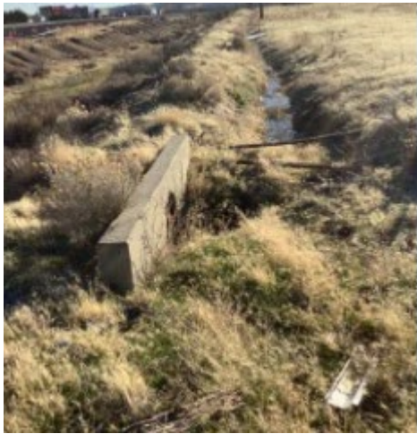
Photograph 17: Concrete foot at conveyance pipe disconnected from upslope pipe. Note minor ditch running to the right of stormwater swale; facing east (Image 0278)
