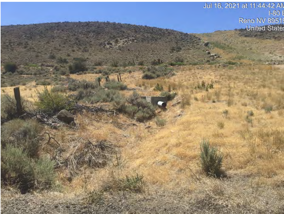
Photograph 106: Drainage piping located near NF-100oad. Photo facing south.
