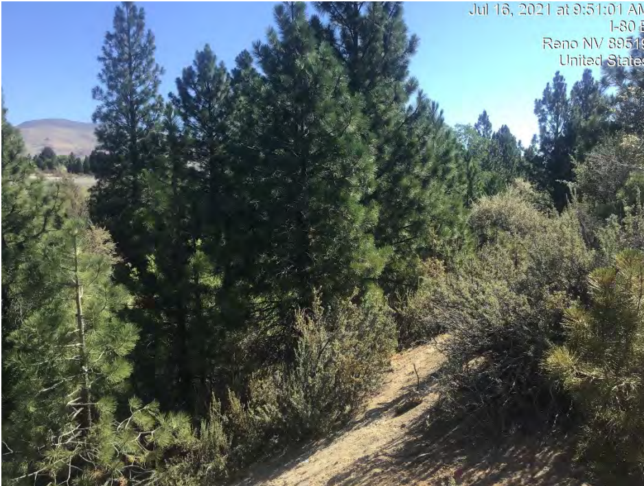
Photograph 57: Dirt embankment incised on ditch. Photo facing northeast. Image 4397 Date: July 16, 2021
