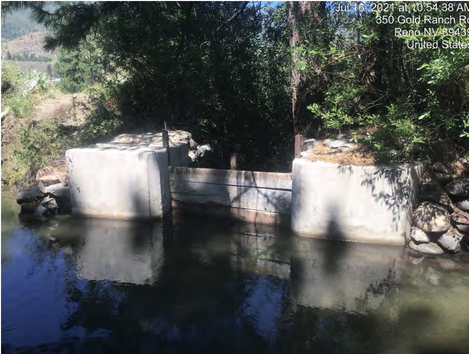
Photograph 97: Culvert with flashboards at the Steamboat Ditch and drainage intersection. Photo facing west. Image 4440 Date: July 16, 2021
