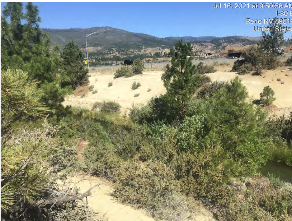
Photograph 56: Dirt embankment incised on ditch. Photo facing northwest. Image 4396 Date: July 16, 2021
