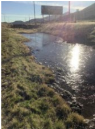
Photograph 7: Standing water in stormwater swale west of 10'x12' access road tunnel under I-80 (Image 0263)
