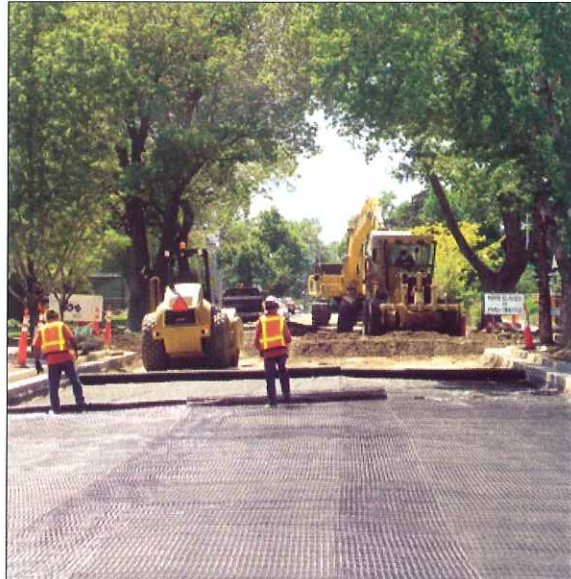
Granite Construction dug up 26 city blocks around the Veterans Medical Center and replaced gutters, sidewalks and roadways during 75 days of construction. Construction crews often helped residents by carrying items to their homes.
